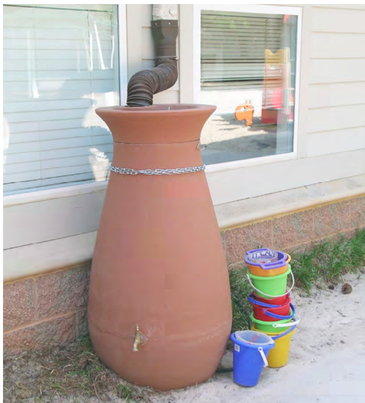
Installed Rain Barrel (has not been elevated)
